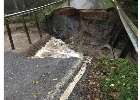
Storm damaged bridge to the eastern part of Orcas Island
